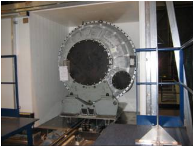
Passive neutron measurement of the uranium hold-up in UF 6 compressors
